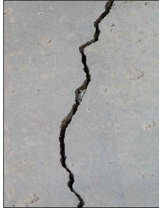
Fig. 4 Close-up View of Example Floor Slab Crack
